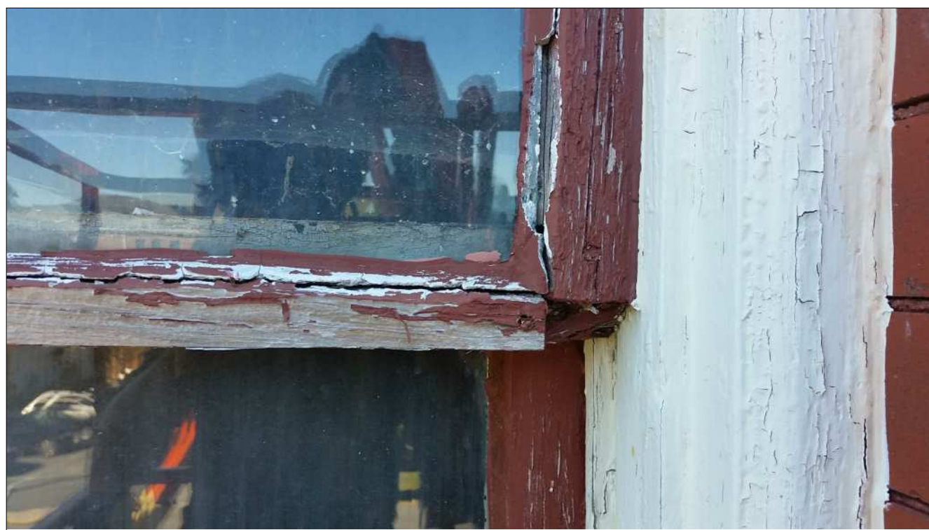
18 TYPICAL FAILING JOINT IN WINDOW SASH TO BE REPAIRED
