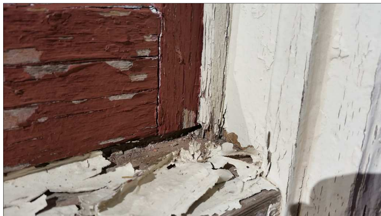
21 TYPICAL DETERIORATED SASHES STOP TO BE REPAIRED AND SOFT WOOD AT WINDOW SASH TO BE TREATED.
