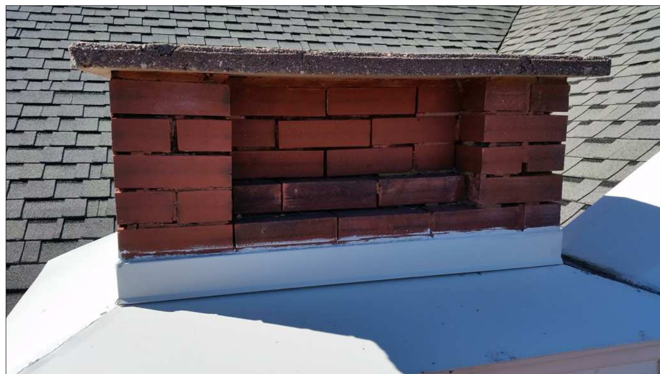
5 TYPICAL CHIMNEY CAP TO BE REMOVED AND REPLACED.
