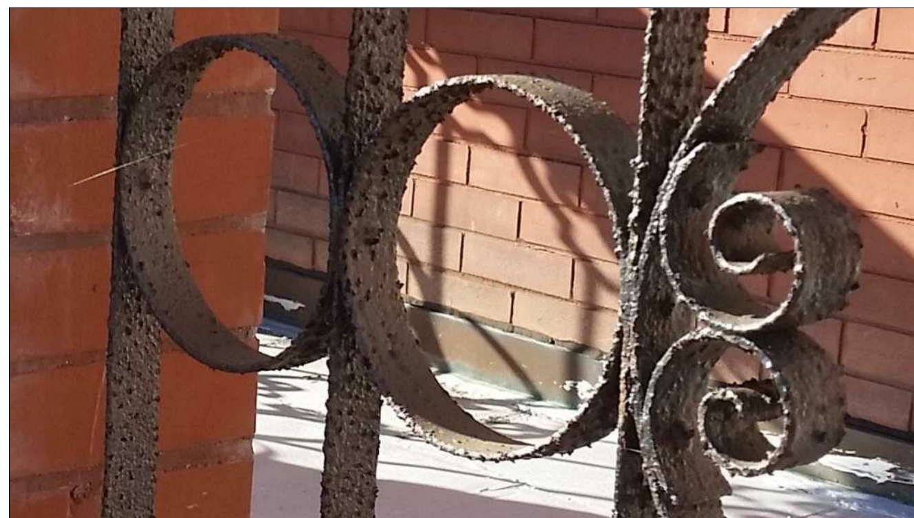
23 IRON WORK TO BE REPAINTED.
