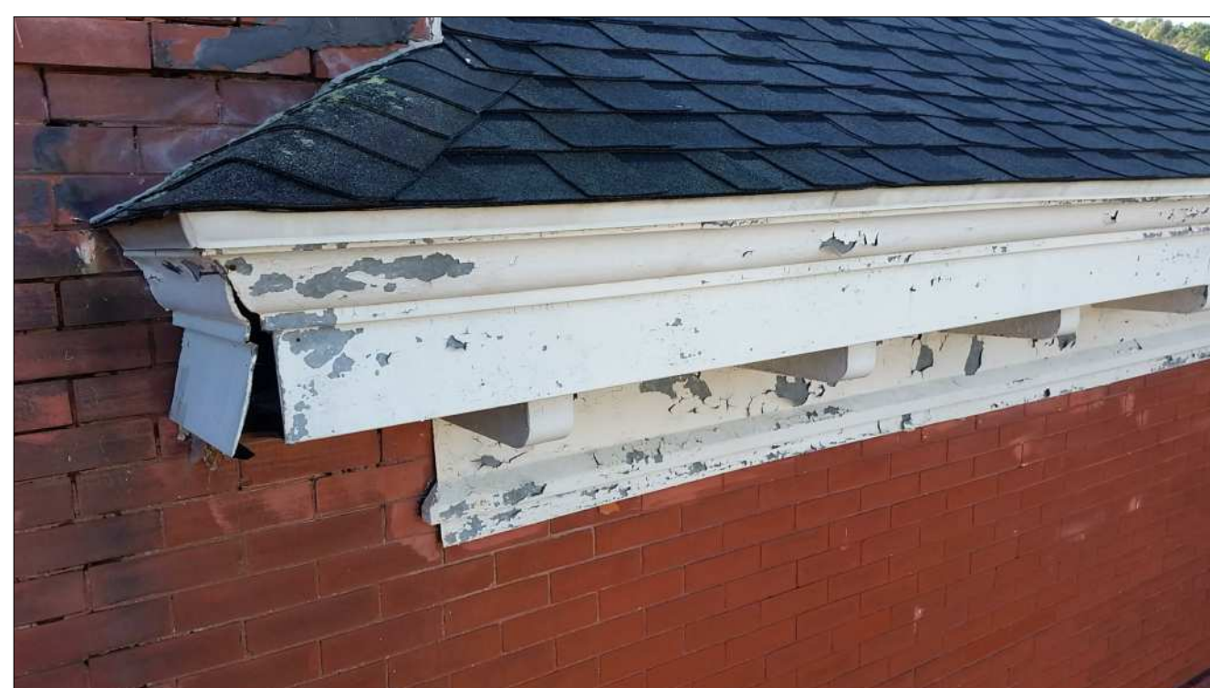
14 TYPICAL FAILED JOINT IN METAL CORNICE TO BE REPAIRED.
