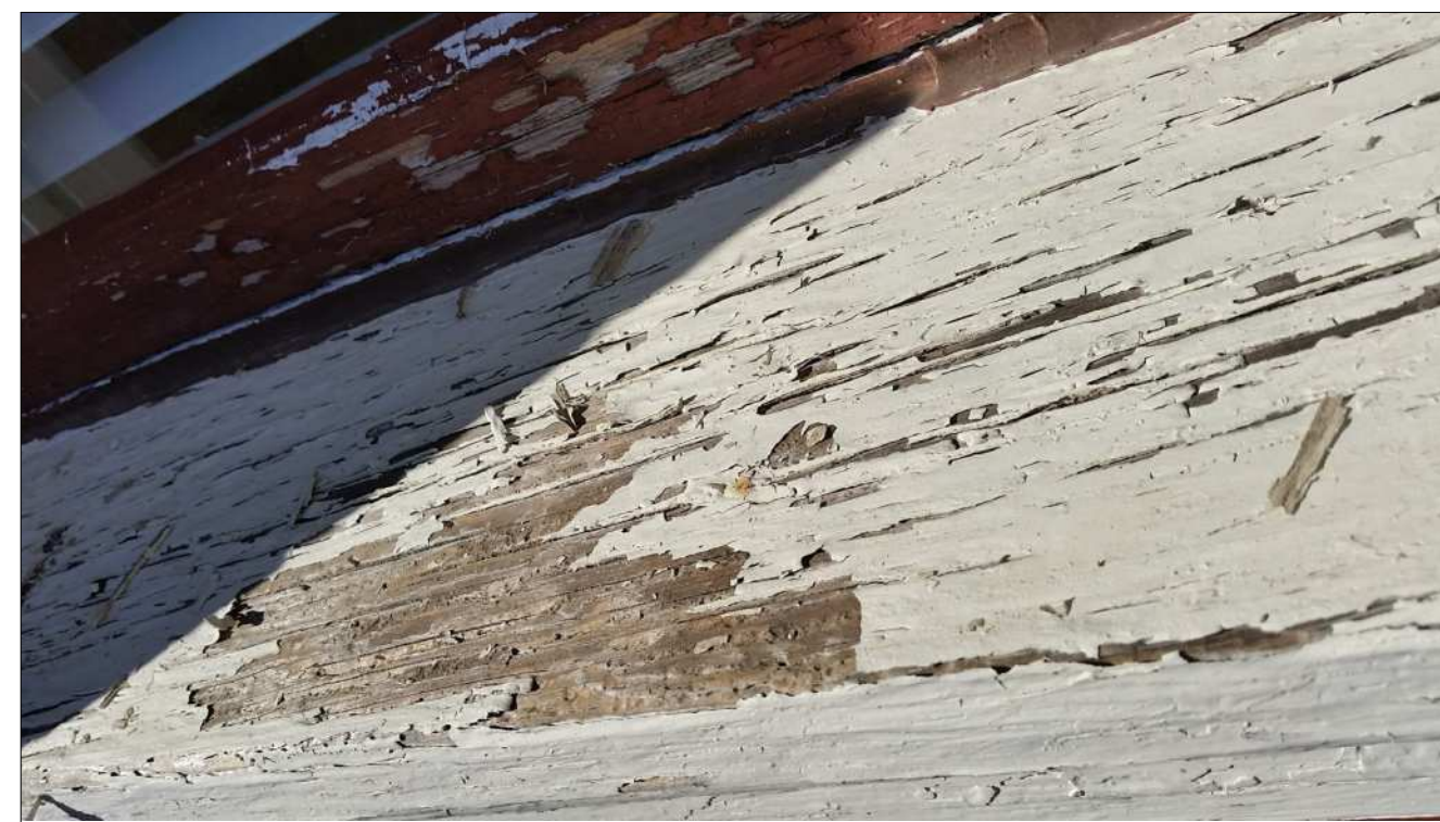
20 TYPICAL CRACKS IN WOOD SILL TO BE REPAIRED.
