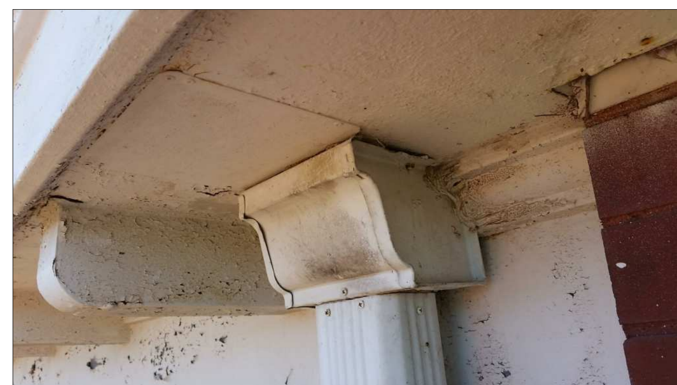
16 TYPICAL DOWNSPOUT TO BE REMOVED AND SOFFIT REPAIRED PRIOR TO INSTALLATION OF NEW DOWNSPOUT.
