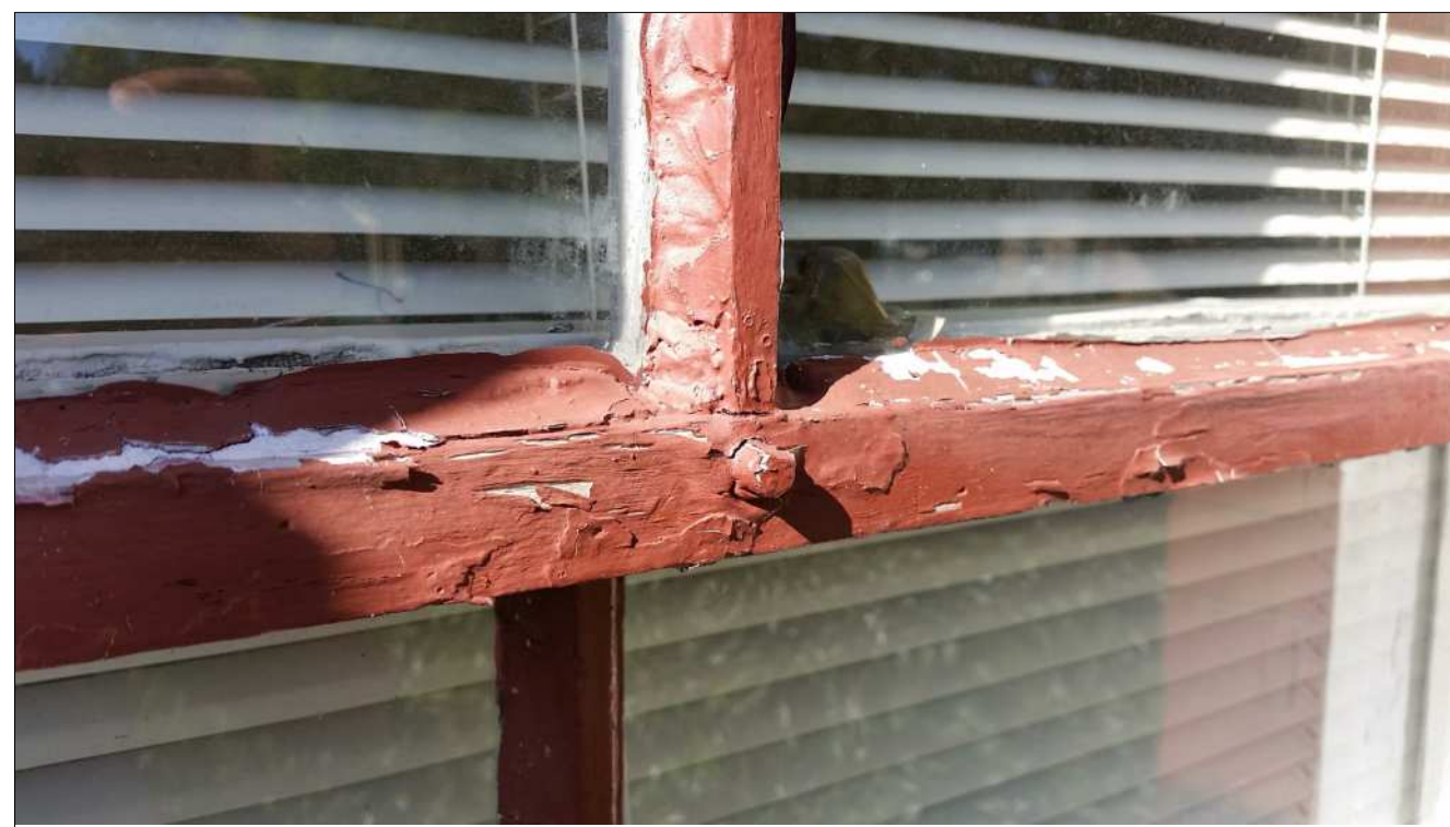
19 TYPICAL PROTRUDING DOWEL TO BE REPAIRED. COAT DOWEL WITH WATER PROOF ADHESIVE AND RESET FLUSH WITH ADJACENT SURFACE. REPLACE DOWEL IF DETERIORATED
