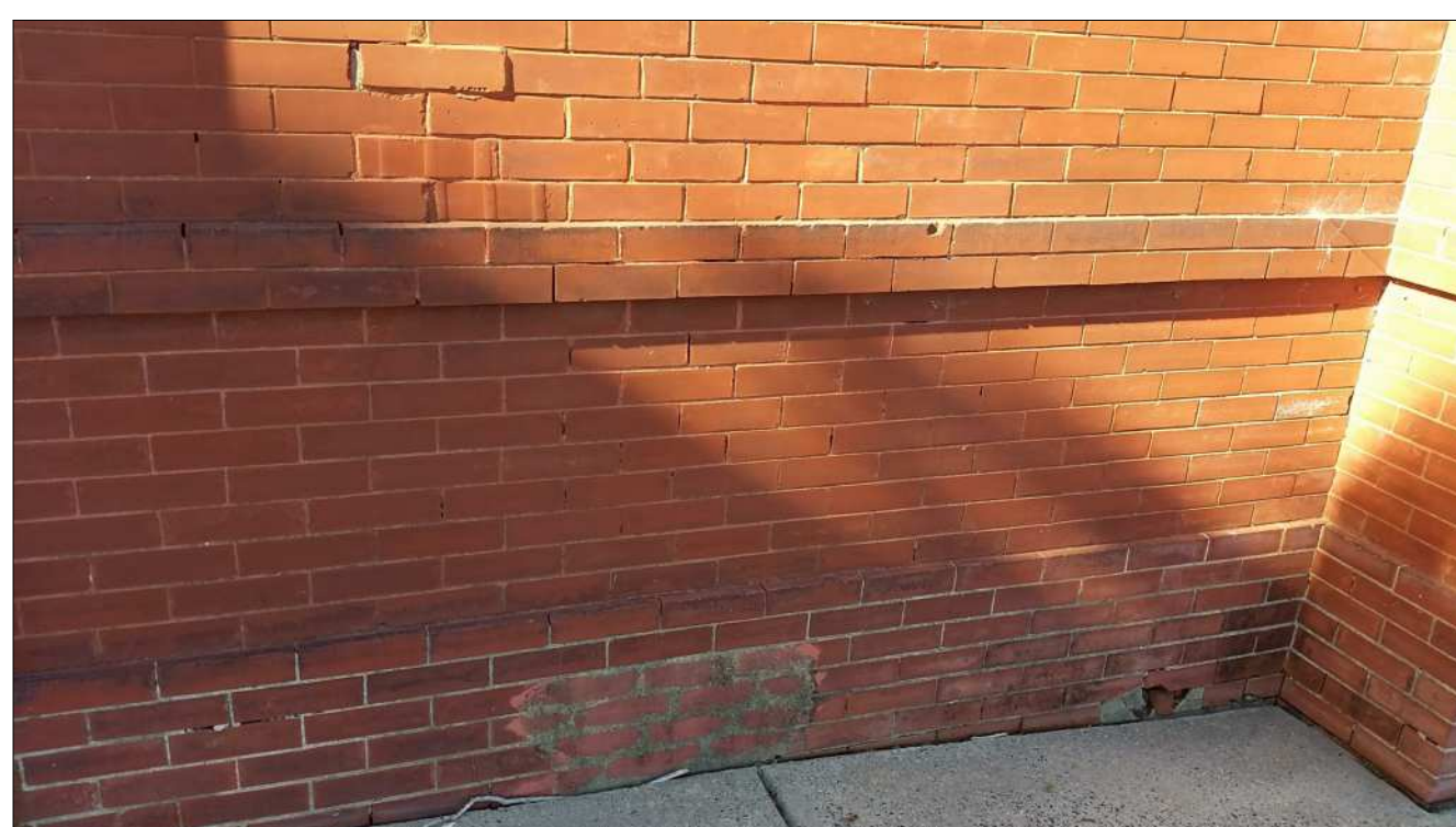
13 TYPICAL MISMATCHED BRICKS USED IN PREVIOUS REPAIR, TO BE REMOVED AND REPLACED.
