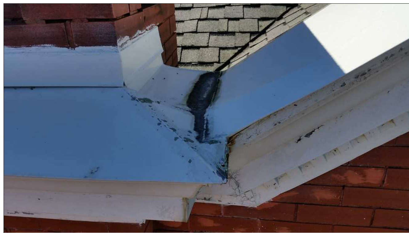
17 PARAPET CAP HOLDING WATER, TO BE REBUILT TO PROVIDE DRAINAGE.
