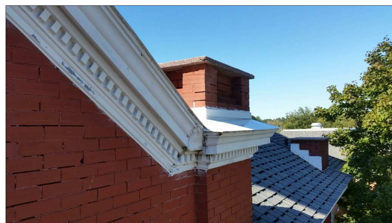
15 TYPICAL JOINT REPAIR WITH INCORRECT PATCHING MATERIALS. REMOVE AND REPAIR METAL TRIM WITH METAL WHICH MATCHES ORIGINAL GAUGE AND PROFILE.
