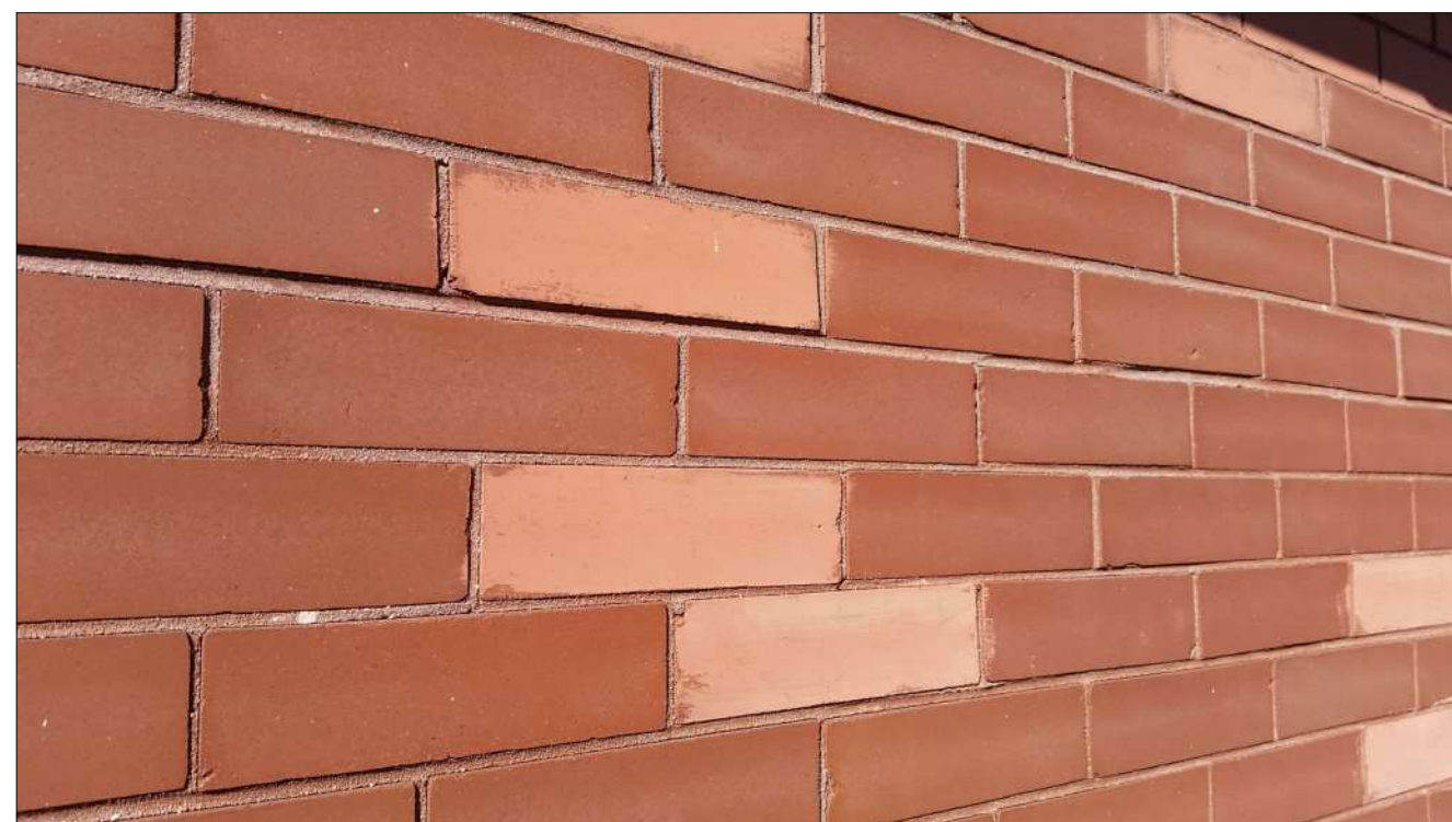
10 TYPICAL PAINT ON BRICKS TO BE REMOVED.
