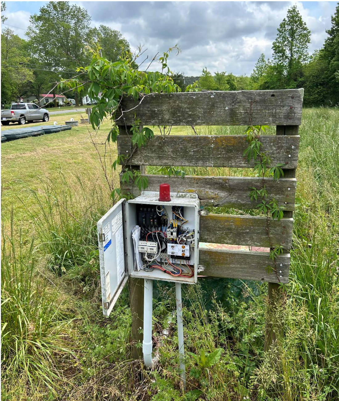
Pump station control panel. Circuits on and pump active.
