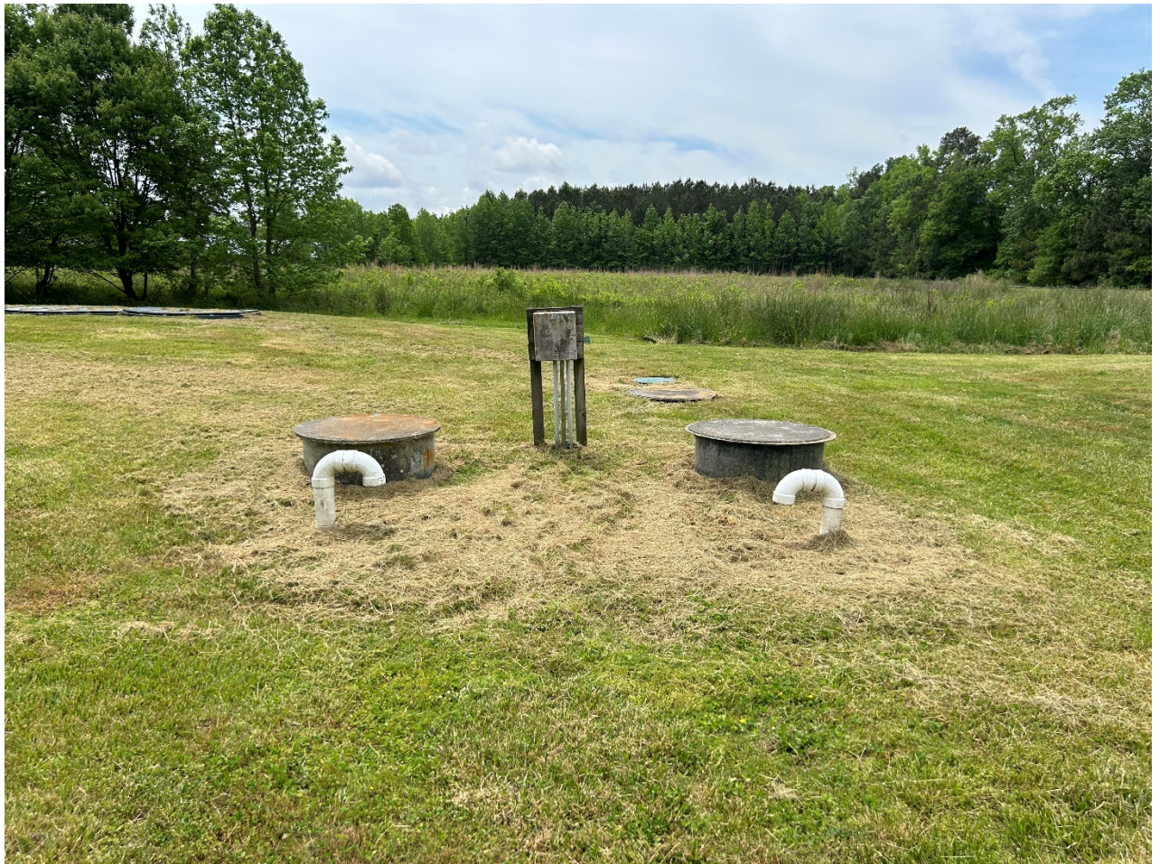
Splitter and pump station. Control panel with circuits on
