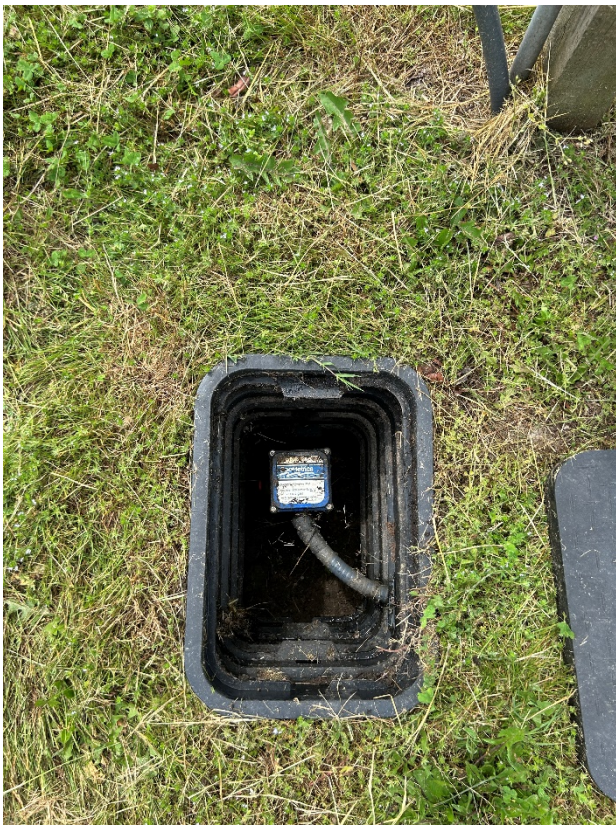
Totalizing flow meter on force main to splitter.
