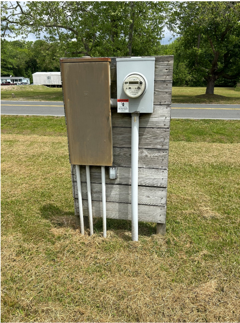
Main power panel.
